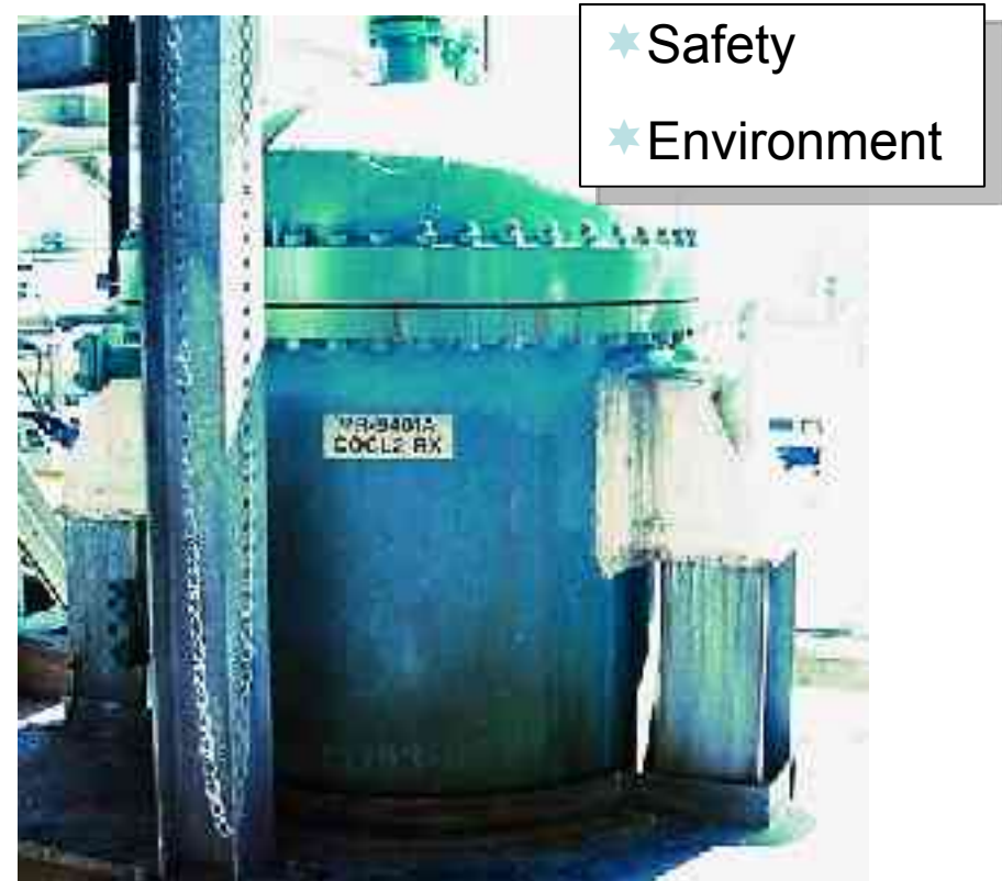
Phosgene Reactor, Geismar, LA
